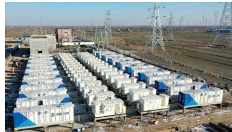
图 8 三峡新能源庆云储能电站航拍图 Fig.8 Aerial photograph of Qingyun energy storage power station, a new energy source for the Three Gorges Project
